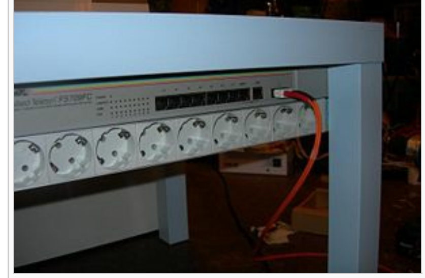
front view: 8 port switch with fiber uplink, and power bar
