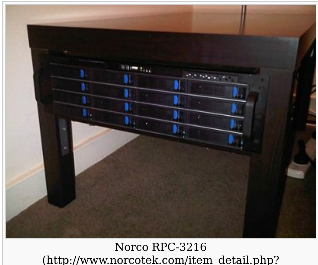
Norco RPC-3216 (http://www.norcotek.com/item_detail.php?categoryid=1&modelno=RPC-3216) mounted in a LackRack Enterprise Edition. Additional brackets used to raise the shelf and support the 45kg+ weight.
