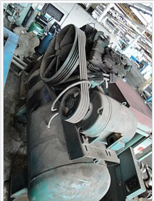
A multiple-V-belt drive on an air compressor
